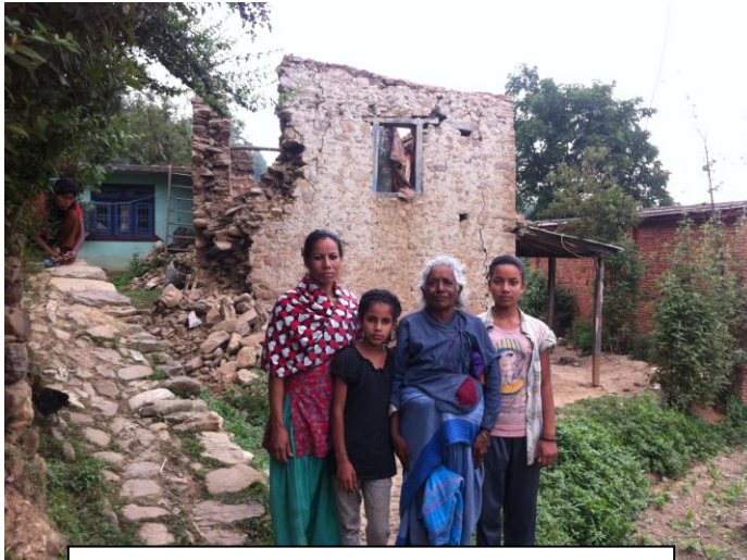
Sunita and Swasthika, with their mother and grandmother standing outside their damaged house.
